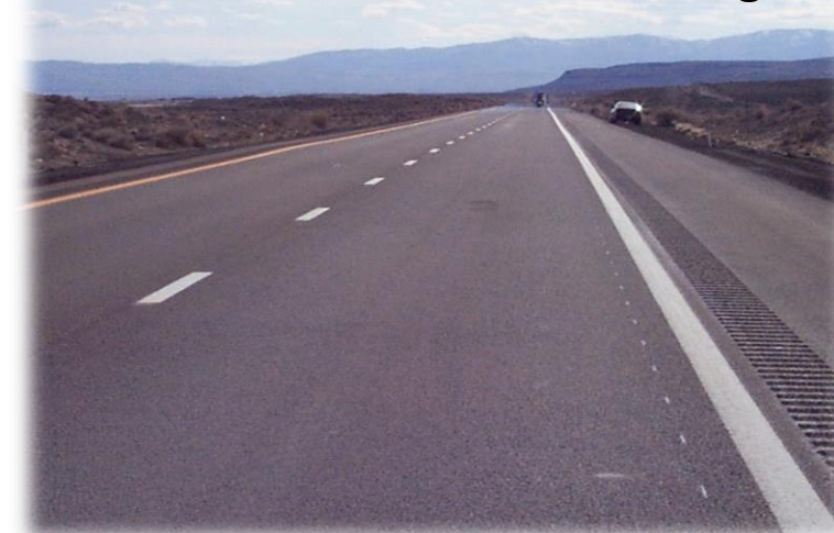
PG 64-22 modified, no rutting
