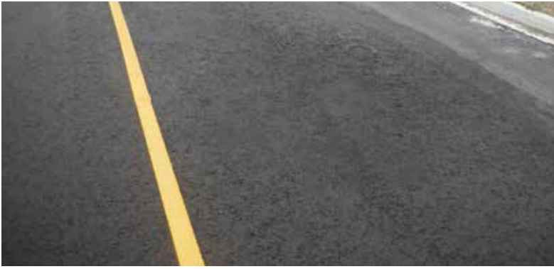
This image shows segregated spots resulting from not having enough head of materials for the auger to spread and/or due to poor workmanship.
